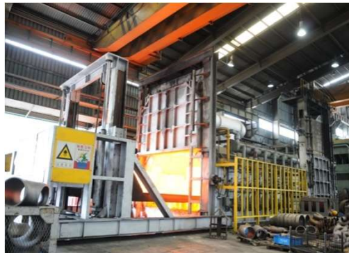
Heat Treatment Furnace For Fitting
